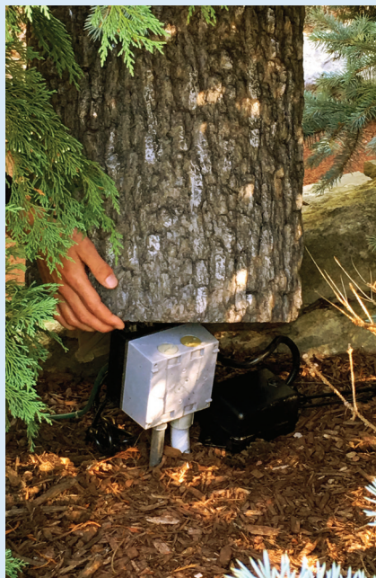
Hide Outlets, Power Cords, and Transformers
